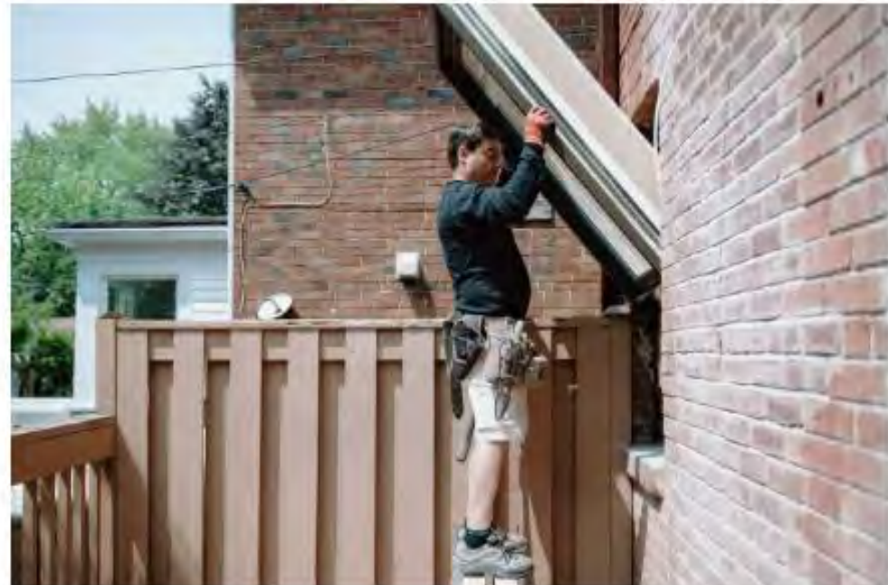
Domenic Masellis installs new windows in a house in Toronto on June 29.
